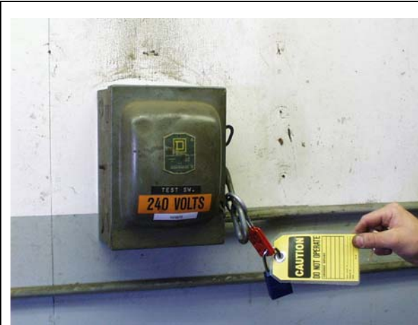
Typical Lockout/Tagout for equipment protection
