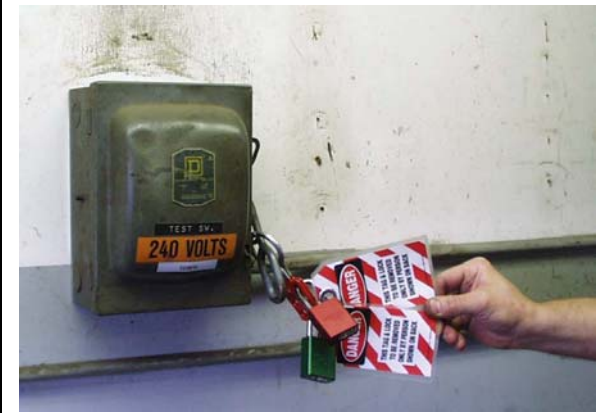
Typical Lockout/Tagout for contractor and personal protection
