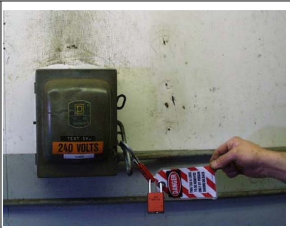
Typical Lockout/Tagout for personal protection
